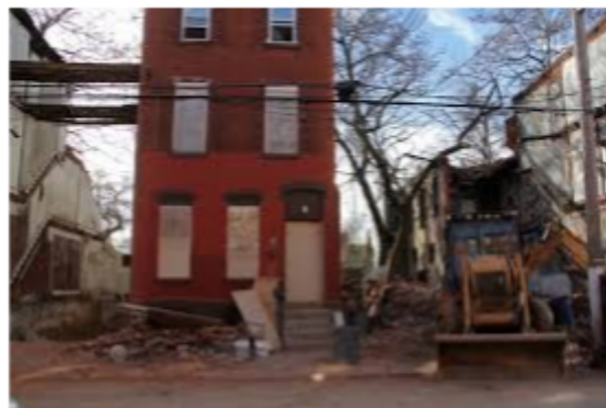
A home is torn down in the Sharswood area of North Philadelphia 31
